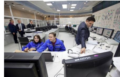
Russia, Rostov NPP Unit 3 - 1000 MW
